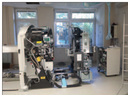
Elektroinstalace gantry PET/CT skeneru
